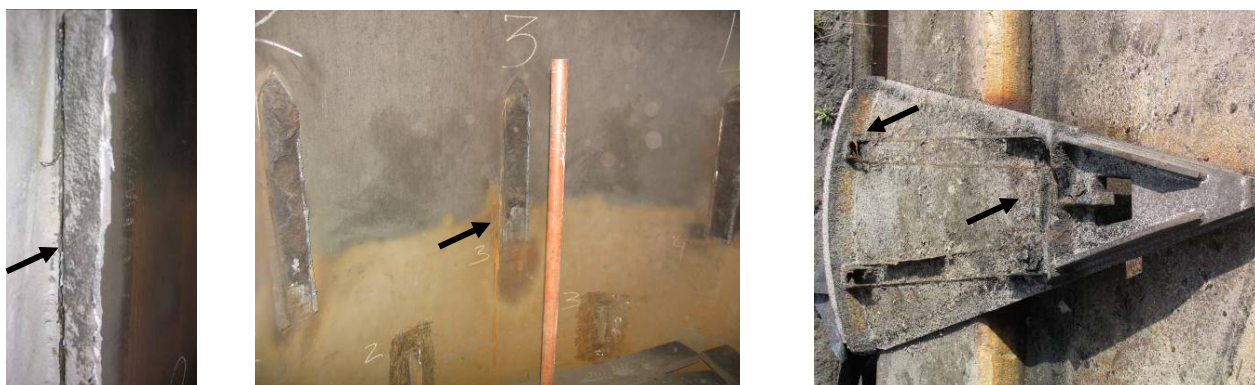
Slika 3. Otkrivene prsline (strelice) Figure 3. Detected cracks (arrows).
