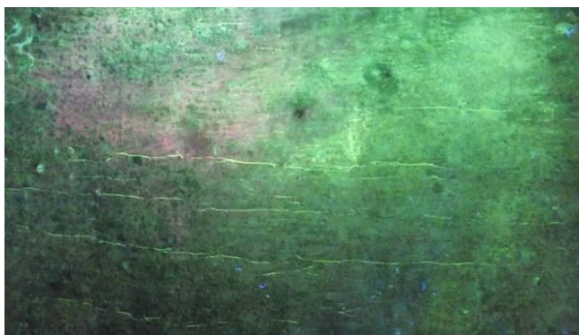
Figure 2. Cracks in base metal observed by magnetic particles, /11/.
