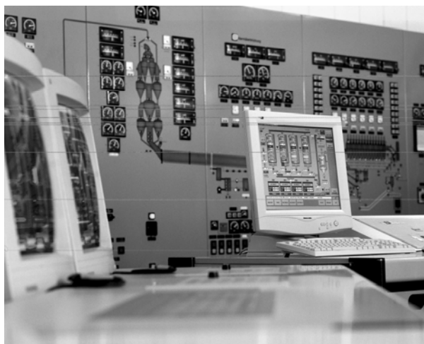
Figure 1 Power station upgraded control room
